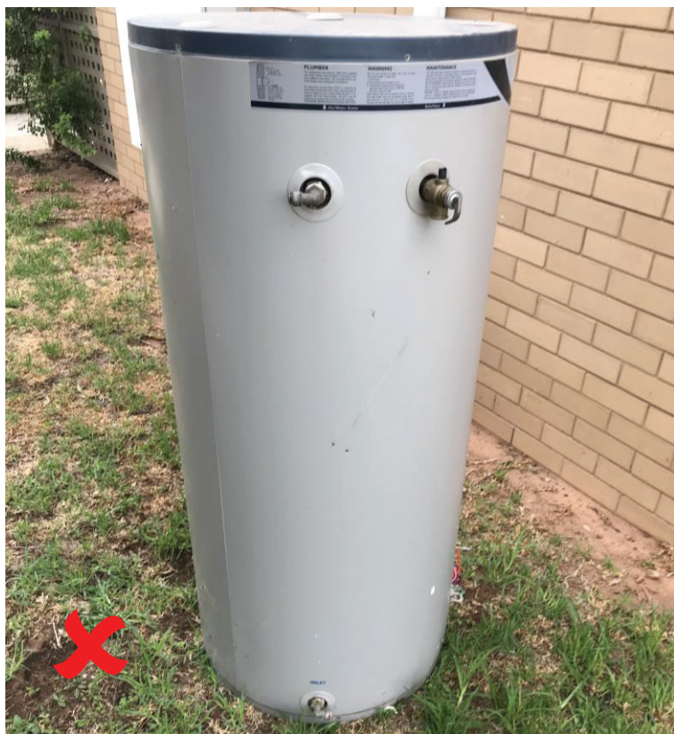
7 Can NOT see method of decommissioning
