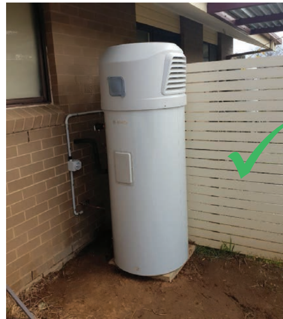
11 Shows full system installed
