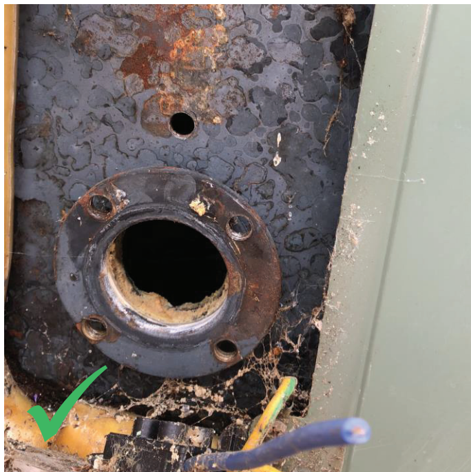
4 Clearly shows hole drilled in tank and element removed
